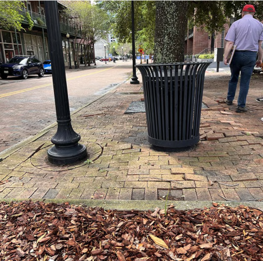
Uneven brick sidewalk
