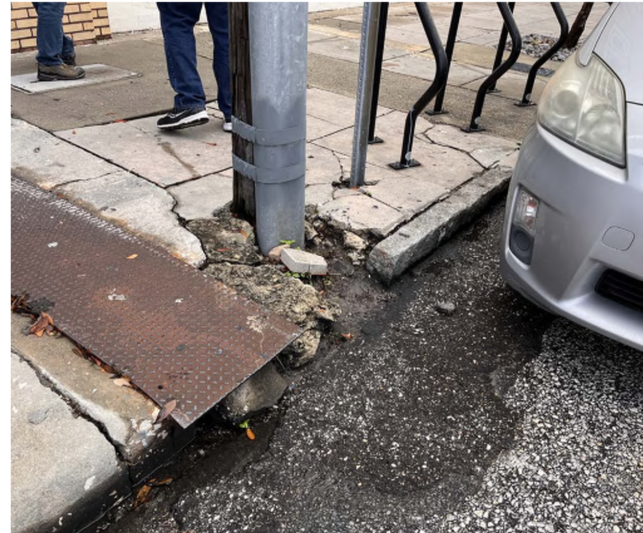
Broken sidewalk and infrastructure issues
