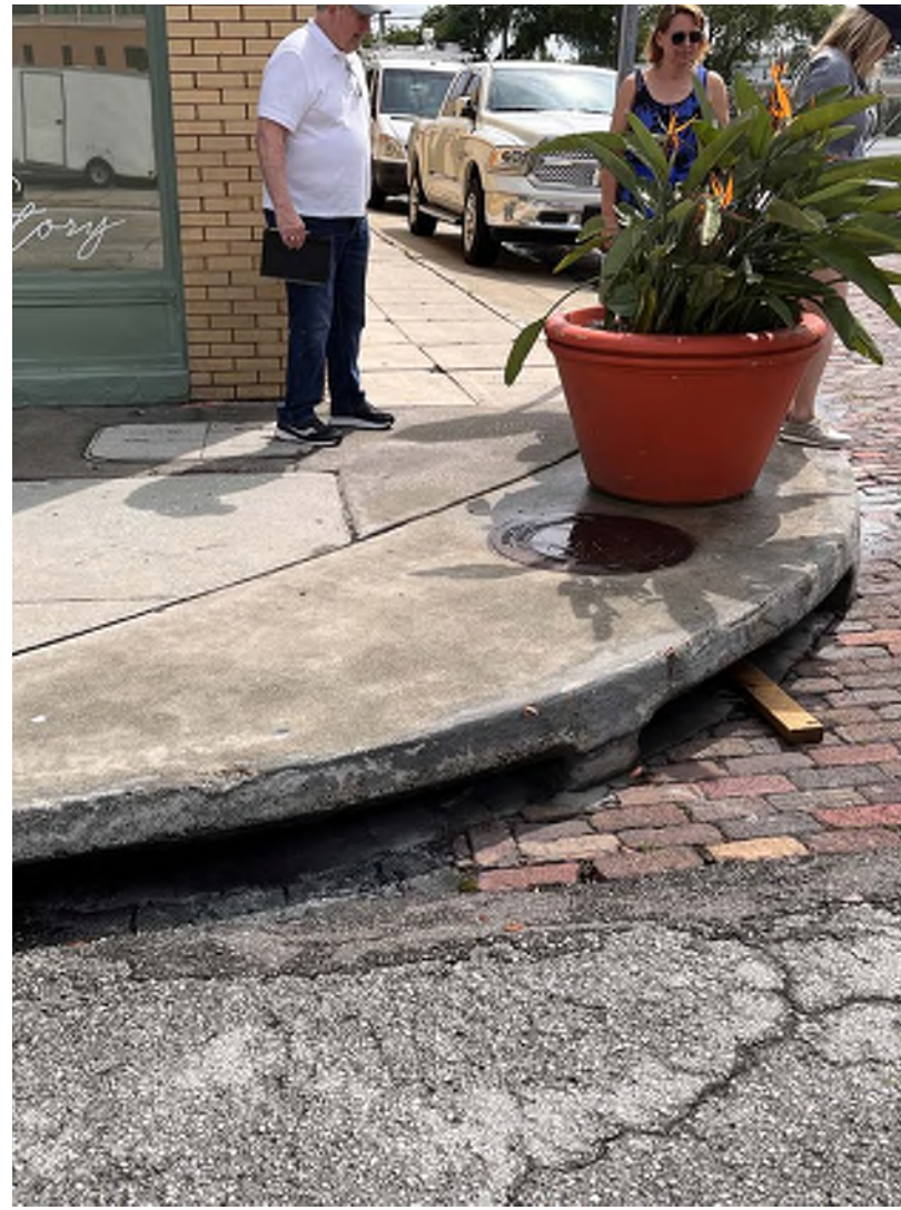
Drainage structure drop-off at street crossing
