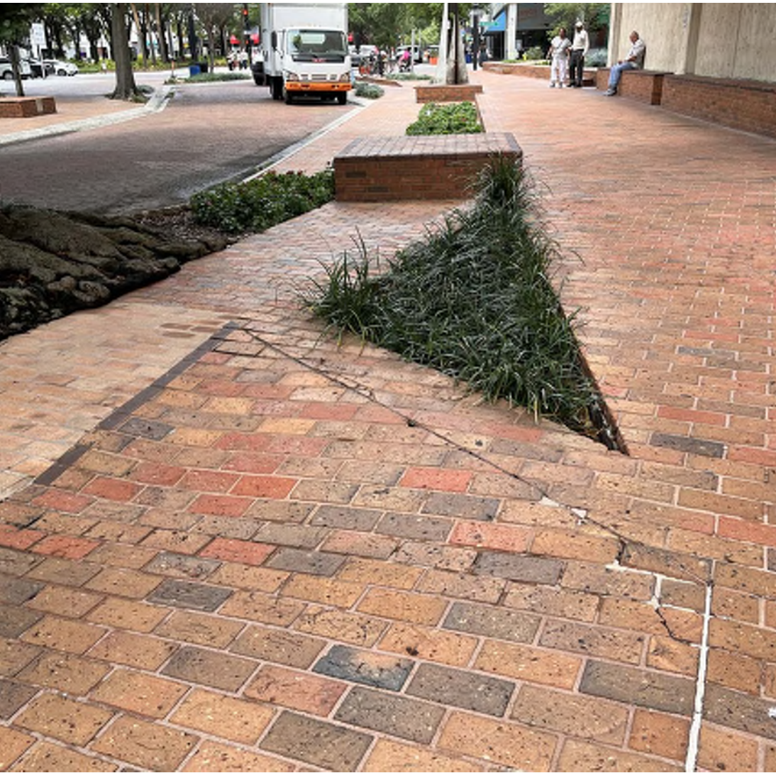
Complicated sidewalk and landscape areas along Franklin Street creating tripping hazards
